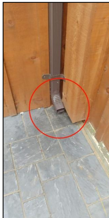
6. Should discharge 6 feet from building
