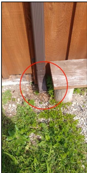
5. Should discharge 6 feet from building
