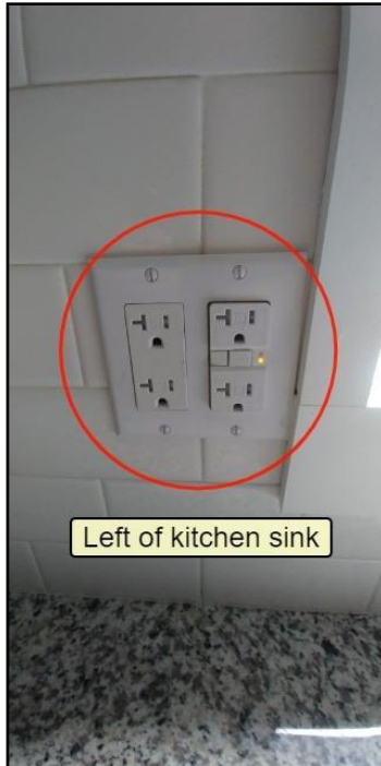
8. Test faulty on GFCI/GFI (Ground Fault...
