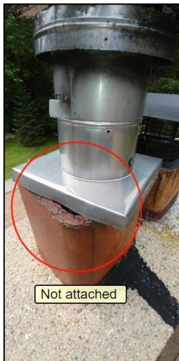
9. Poor connection to chimney
