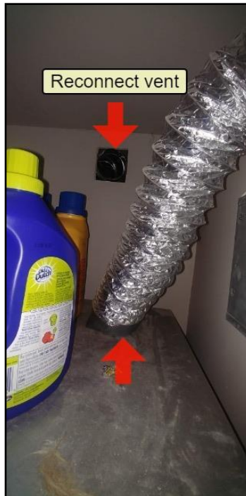
15. Not vented to exterior
